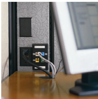
Above Work Surface Electrical
